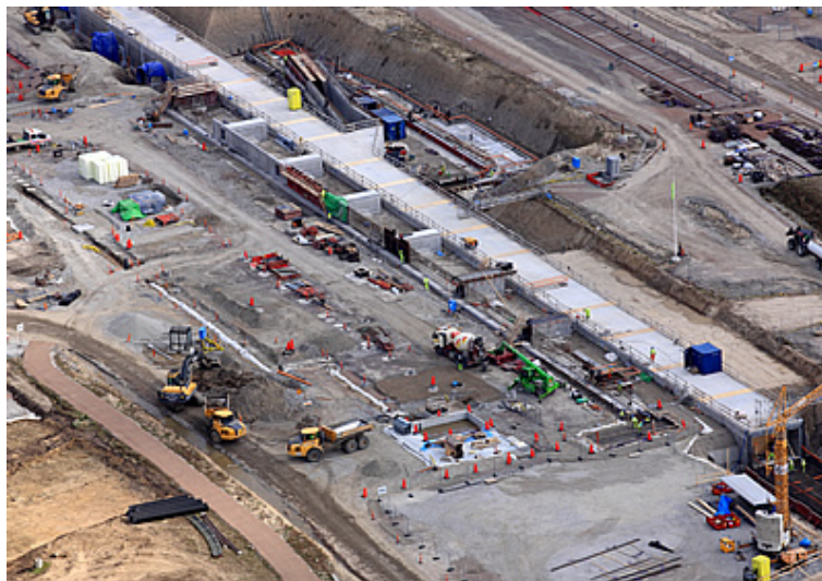
Aerial photo of the ESS Accelerator tunnel and Gallery Building under construction on 18 September 2015. PHOTO: Perry Nordeng
